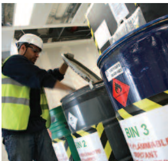
Facilities for hazardous waste are provided on each floor and are emptied at the end of each day, reducing potential risks for workers.
